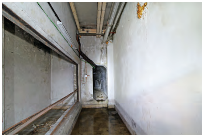
The filter room with the emergency escape tunnel on the far side
